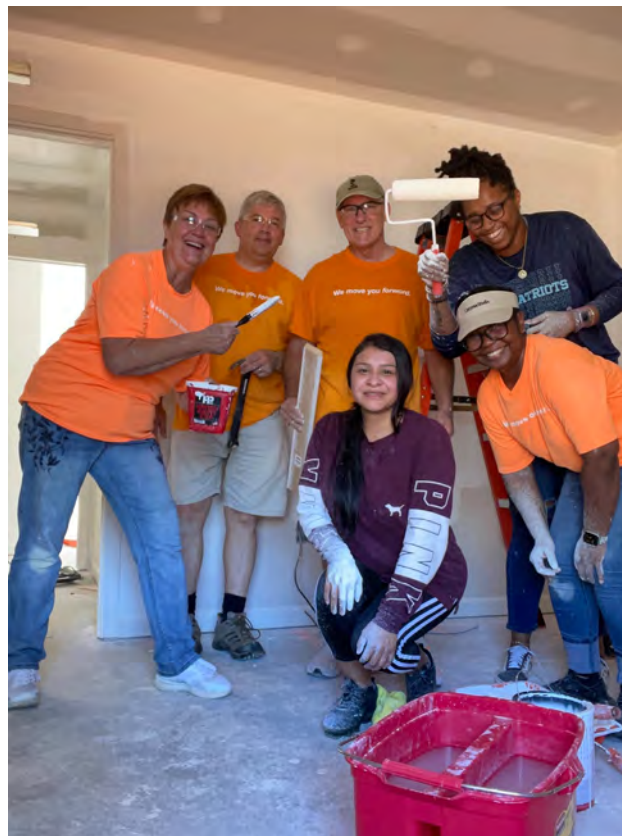
Carolina Foothills FCU staffers take part in a Habitat For Humanity home-building event.
